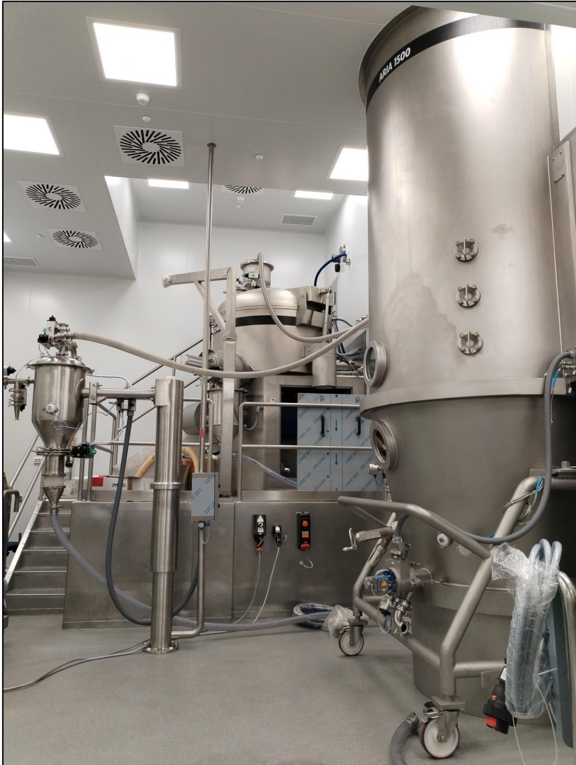
Aria and Rotomix 1500 located in Granulation Room 1
